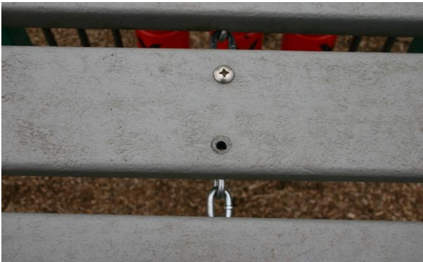
Metal Composite Structure- Suspension Bridge- Outer Chains Rusted- MAINTENANCE
