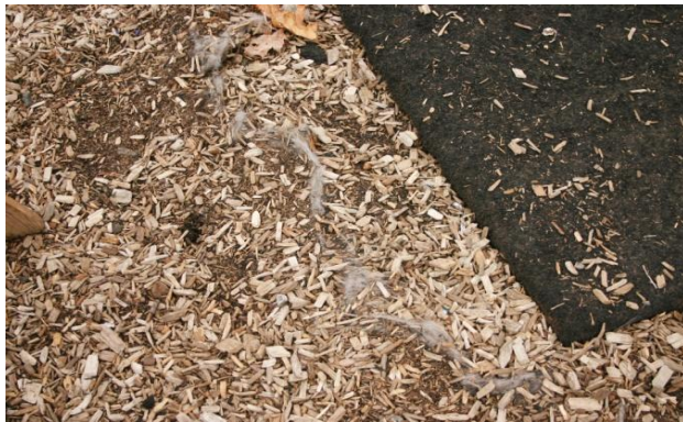
8ft Swing Set- Fabric exposed - Class B Hazard
